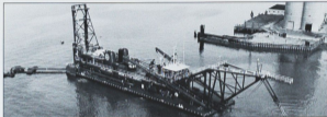
The hydraulic dredge is excavating a trench in the harbor bottom for the tunnel.
