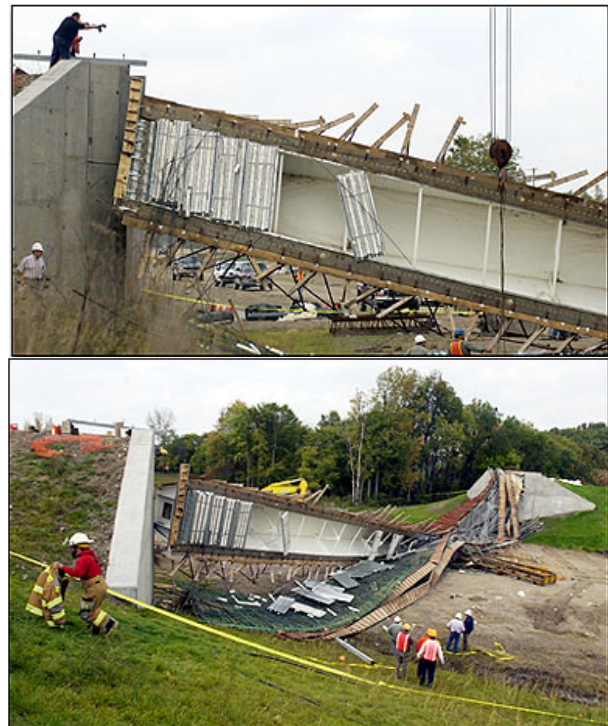
Figure 1: Marcy Bridge collapse [5]
