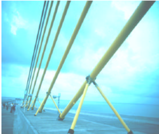
Figure 2: Sunshine Skyway Bridge Dampers
